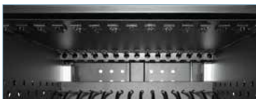
Each shelf includes clips and wire routes to avoid cables tangling or falling behind the shelf
